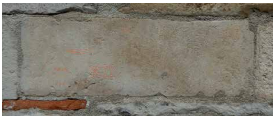
Fig. 7. Bloc with graffiti (So3) from the southern wall with graffiti enhanced. Photo E. Hobdari
